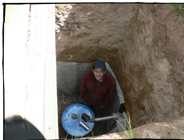
Where I'm sent when I get in trouble, or else our grey water drainage system installed this summer
