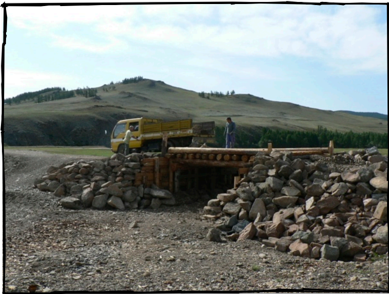
Building a new bridge on the road to one of our fields
